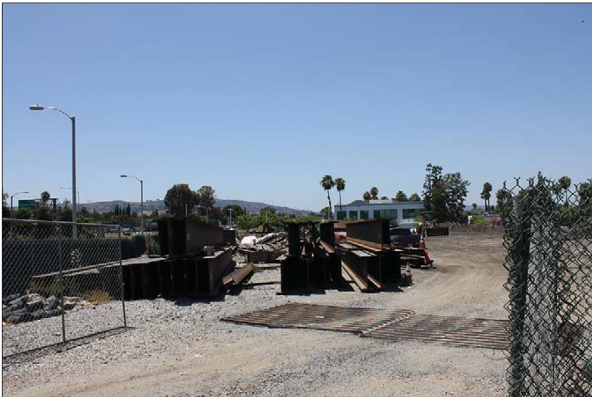
Photograph 3: ACE Nogales Street Grade Separation Project construction laydown yard, southwest corner of Project Site
