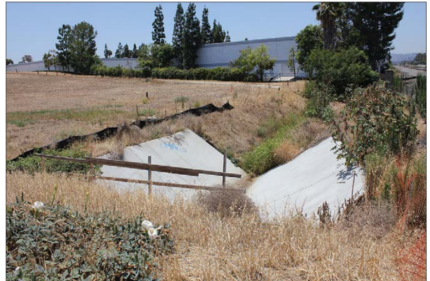
Photograph 4: Looking west along partially channelized storm drain, north end of Project Site
