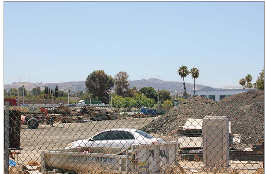
Photograph 4: ACE Nogales Street Grade Separation Project construction laydown yard, southwest corner of Project Site
